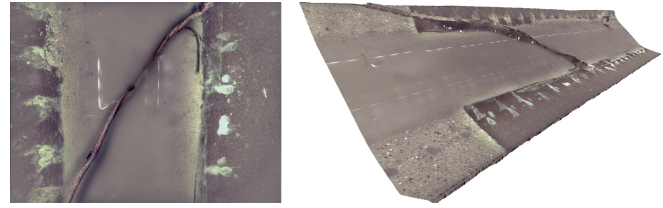
Fig. 1: Pipeline DN 400, stoneware, example based on root load in the bottom of the pipe (left individual texture image, right stitched RGB-D pipe section) at travel speed 10 cm/s
