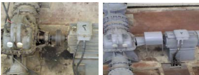
Guarding of pump/motor coupling, Dishna WTP, Qena, Upper Egypt
