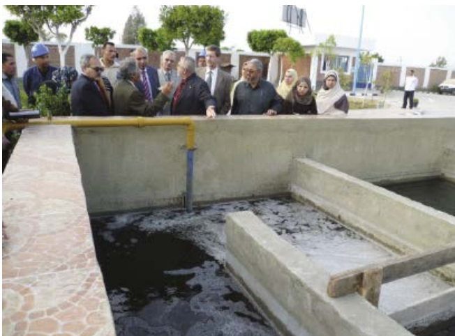
TSM Egypt site inspection of the Chlorine Contact tank at Hehia WWTP, Sharkia Governorate, Nile Delta
