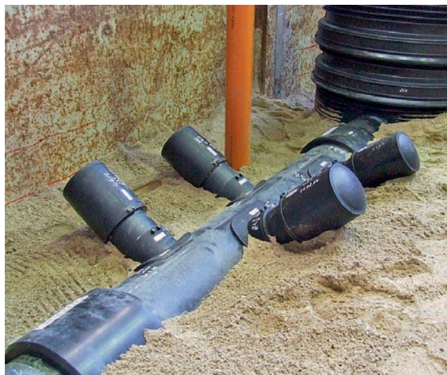
Fig. 16: Detail of the test set-up with four FRIAFIT sewage saddles before burying
