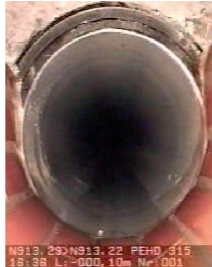
Fig. 12: Camera inspection in the area of the man whole connection and transition from clinker-clad channel to PE pipe
