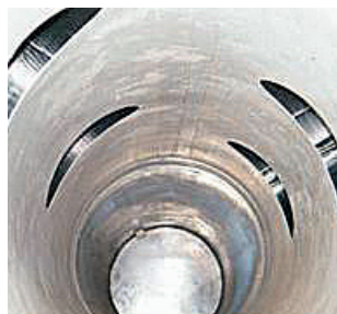
Fig. 15: View into the sewage pipe: smooth, displacement-free inlets, good inspection capability of the pipes thanks to bright interior coat
